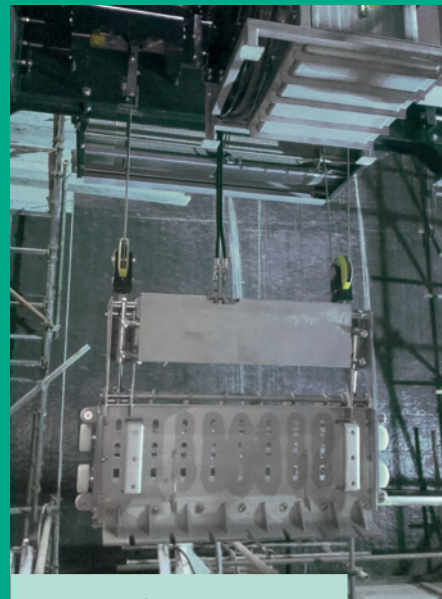
Trash Rack Screen in use
