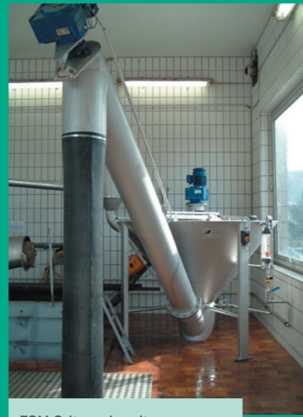
FSM Grit wash unit
