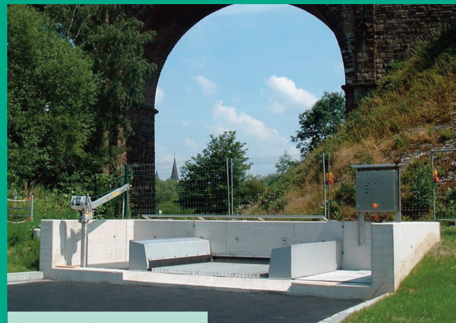
Grit Receiving Station
